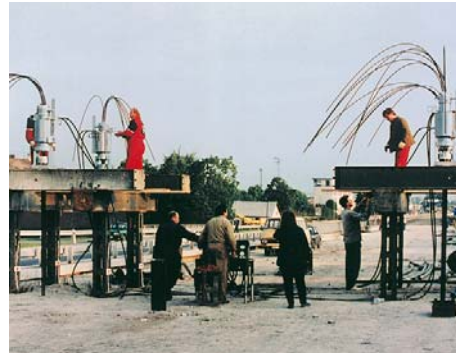
Fig. 16: TENSAM 3000 kN stressing jack used for the reconstruction of a motorway – lifting of sections for repairing the bearings
